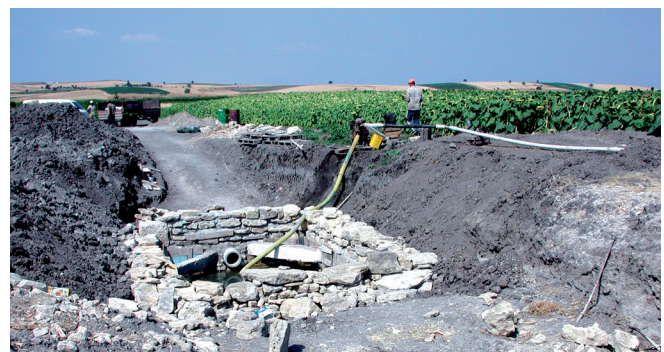
Fig. 17 Looking to the north from near the west of Alacalığöl mound (the mound is just to the right of the photograph). Owner of the field dug a deep well to collect excessive ground water and drain to main drainage ditch to the north (See Figs. 2, 13 and 14). The mouth of drainage pipe to empty the well is seen on the wall. Because of deposition in the Alacalığöl swampy environment, color of the earth is black.
