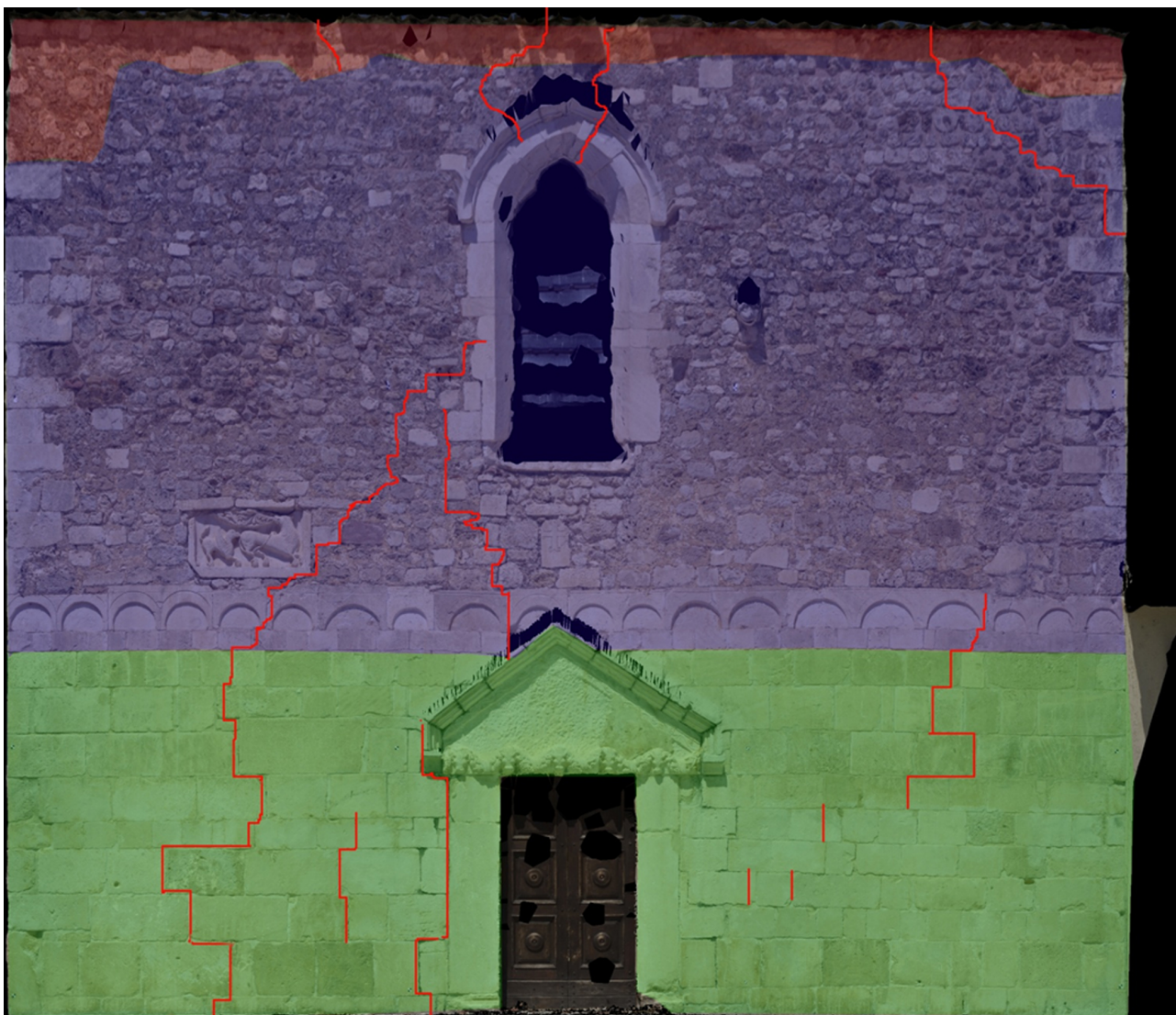
Figure 8: Orthophoto of the façade with lesions and main building phases of the Church of San Pietro, Coppito (AQ).
