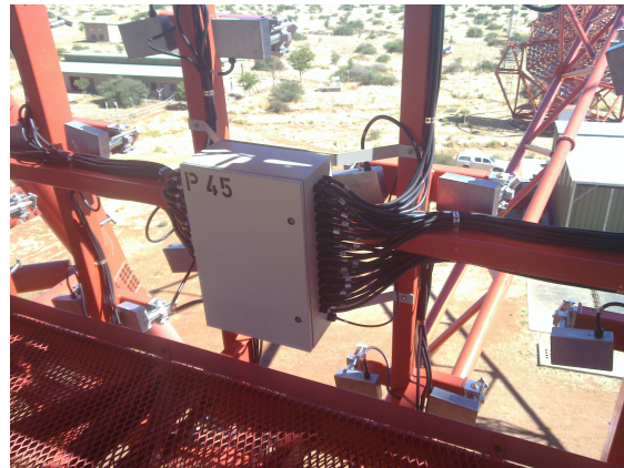
Figure 6.13: A panel controller box in CT5. Power and signal cables connect up to 84 motors with each box. One optical cable leads to the central box.
