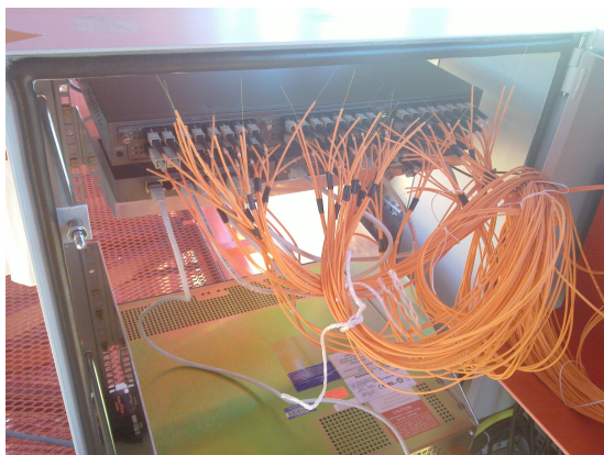
Figure 6.10: The media converter in the central box and the optical fibres coming from the panel controller boxes.
