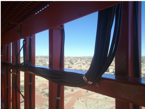
Figure 6.12: Power cables in CT5. Metal stripes are screwed to the steel structure to fixate the cables.
